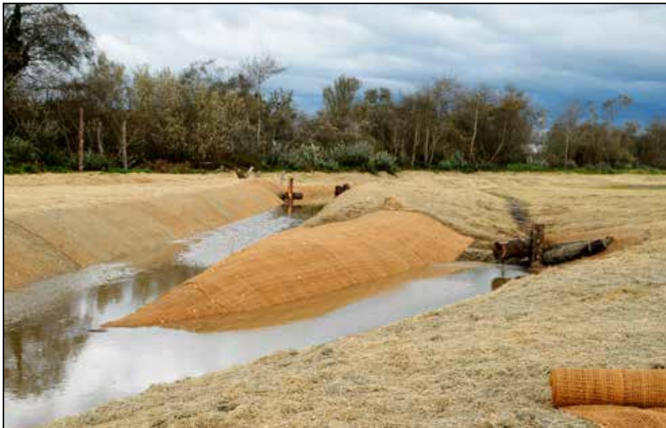
A nearly completed portion of the Salt River Restoration, waiting for tree and shrub plantings. Main channel on the left, active berm in the middle, and floodplain outlet on the right with large woody debris structures.
