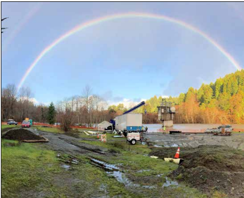
Humboldt Bay Municipal Water District (HBMWD) Collector 1 and 1A Rehabilitation Project. Mad River, Arcata, California. Completion 2017.
