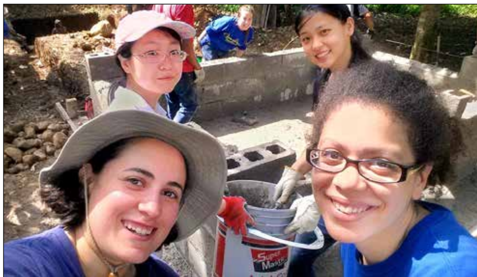
Margarita Otero-Diaz (bottom left) helping to construct a pedestrian footbridge in the rural community of Vaquilla, Panama, in August 2015. The project was through the student group Bridges to Prosperity.
