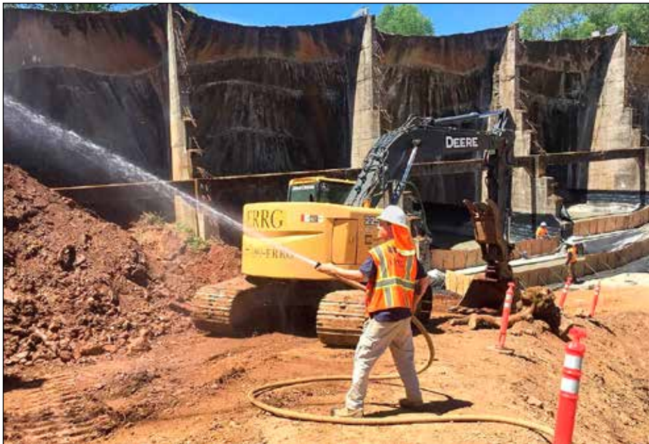
Steven Hopper on the firehose at the Argonaut Mine sediment dam near Jackson, California. Dust suppression minimizes the spread of arsenic.
