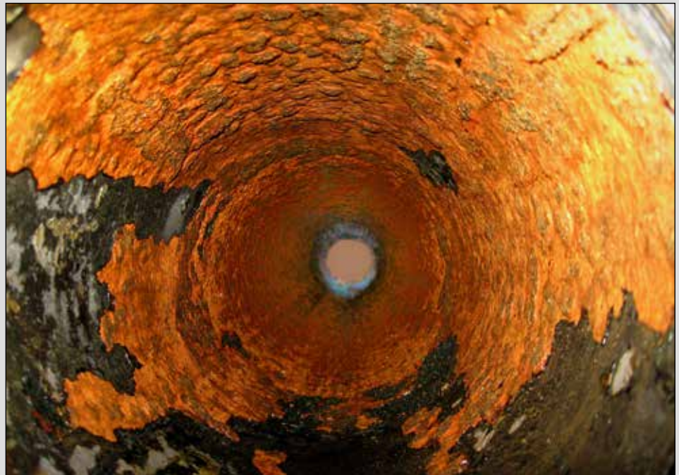
Humboldt Community Services District's South Bay Well corroded casing. HCS D is currently replacing the well as part of its on-going infrastructure replacement program.
